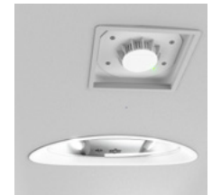
New Smoke Detector
